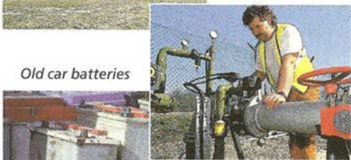
Recycling methane from a landfill site
